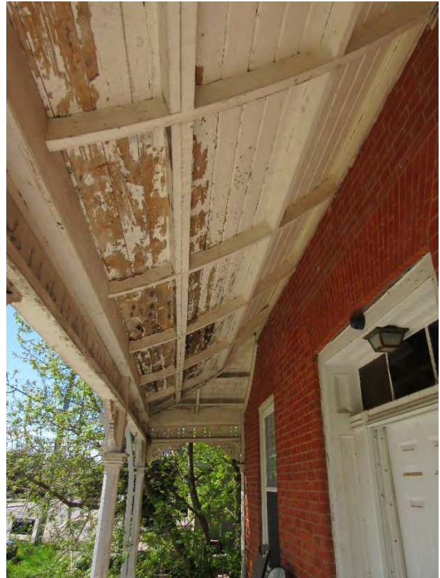
Figure 49: Underside of porch roof with peeling paint on wood
