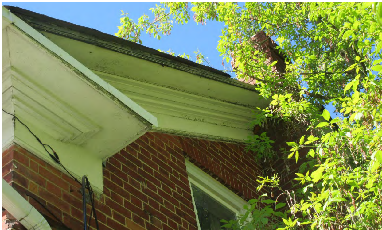
Figure 46: Fascia and soffits at roofline along north with wood return at far left
