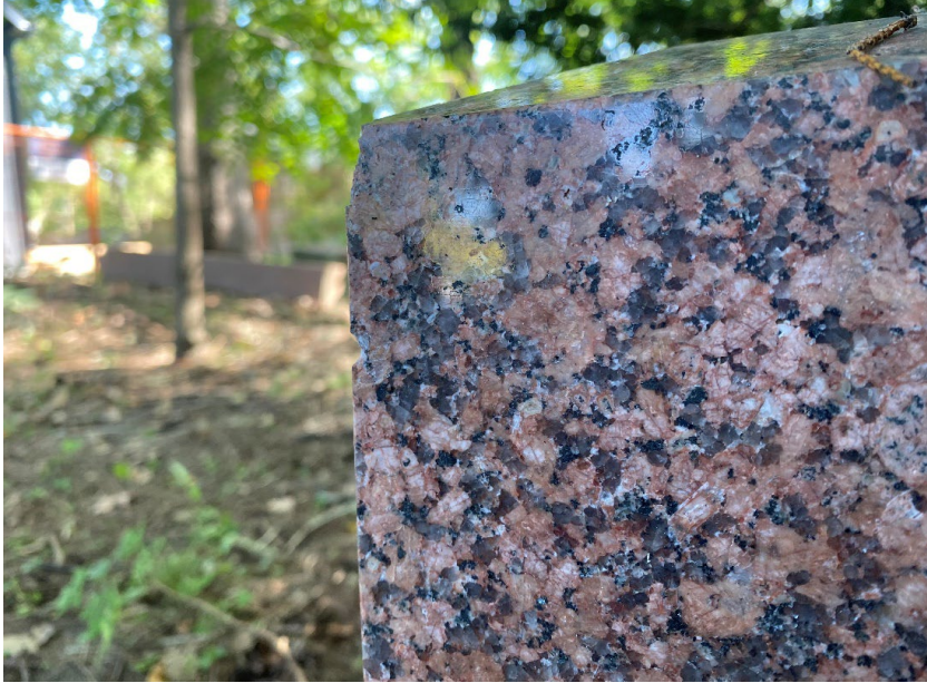
Figure 42: J16-1 chipped corner on middle stone from machinery (A.S.I., 2023).
