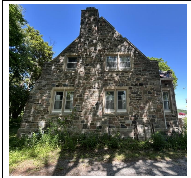
Photo #2: West facing elevation of gatehouse. Staff note the damaged ridge cap along the gable.
