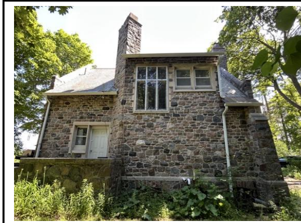
Photo #3: North facing elevation of gatehouse. Staff note the windows and door are not original to the structure. Staff also note missing slate shingles on the west side of roof.
