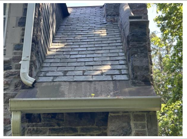
Photo #6: A closer photo of the missing shingles also seen in Photo 3. Staff note the deterioration of remaining shingles.
