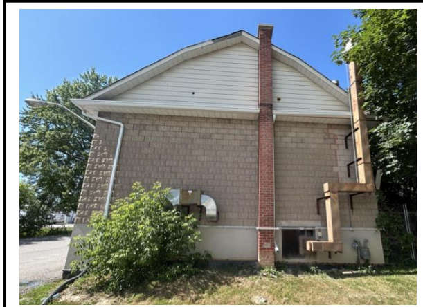
Photo #3: South facing elevation of Nobleton Community Hall. Staff note the existing ventilation ducting is proposed to be removed/relocated.
