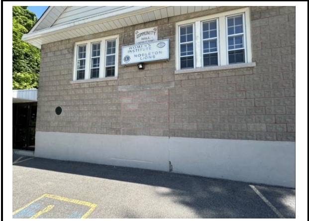
Photo #4: Closer photograph of North facing façade. Staff note damaged portions of the façade that are proposed to be restored.
