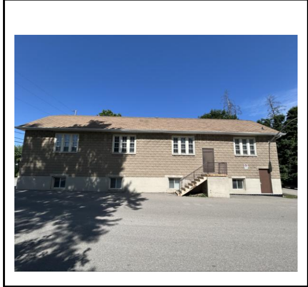
Photo #2: West facing elevation of Nobleton Community Hall. Staff note the staircase and doorway shown in this image are proposed to be replaced and enlarged, respectfully.
