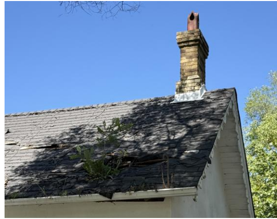
Photo #6: A closer photo of the hole in the roof, also seen in Photo 1. Staff note the deterioration of the remaining shingles and the vegetative growth.
