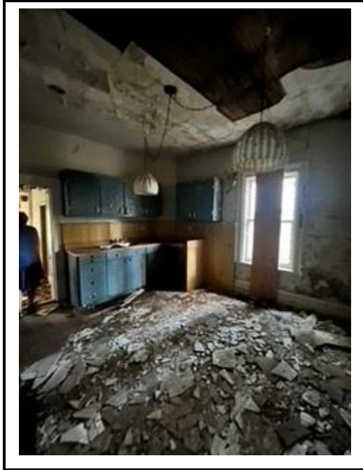
Photo #8: Images of the interior provided by the applicant. Staff did not enter the structure due to safety concerns.
