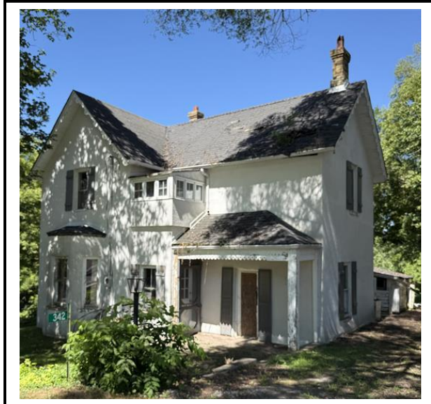
Photo #1: South facing elevation of subject structure. Staff note the damaged roof, in which a hole is visible beneath the east chimney. Staff also note the rotting/decaying shingles.
