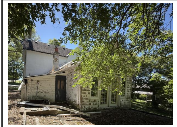
Photo #3: North facing elevation of subject structure. Staff note extensive deterioration of the rear addition.
