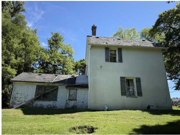
Photo #5: West facing elevation of the subject structure. Staff note the deterioration of the rear addition, including the roof and its elements.
