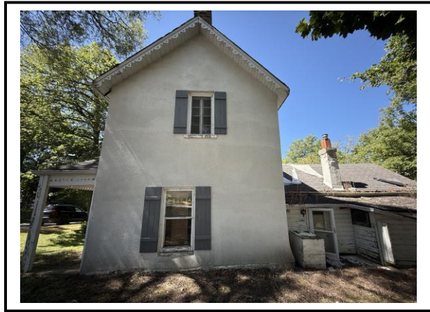
Photo #2: East facing elevation of subject structure. Staff note the rotting/decaying state of the window frames and sills.
