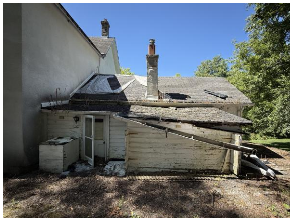
Photo #7: Closer image of east elevation of rear addition. Staff note the significant deterioration and damage to this element of the structure.
