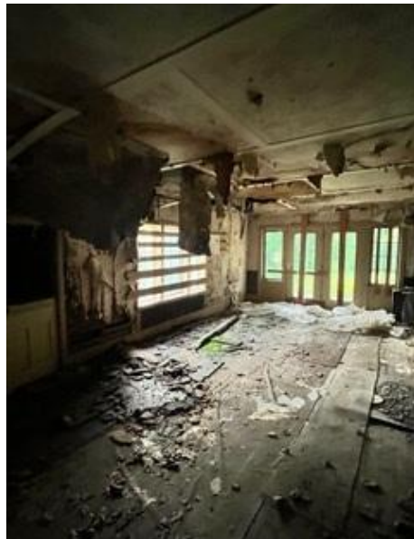
Photo #8: Images of the interior provided by the applicant. Staff did not enter the structure due to safety concerns.
