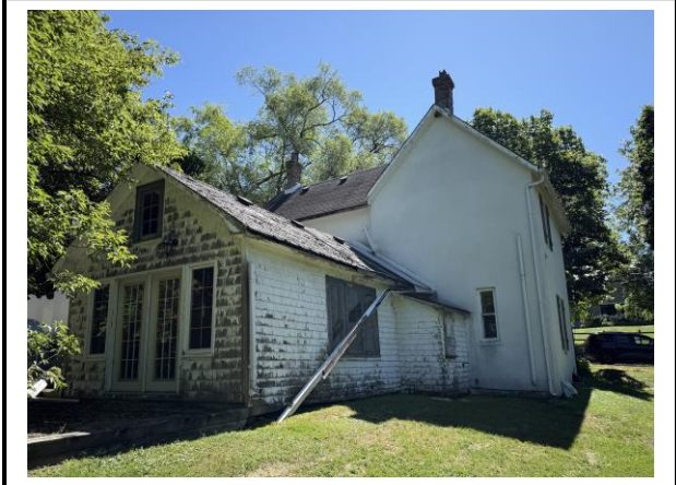
Photo #4: West facing elevation of subject structure. Staff note extensive deterioration of the rear addition.
