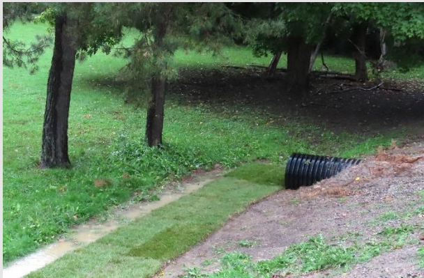
Drainage from Snowberry & Kingscross Water from Thursday's rain
