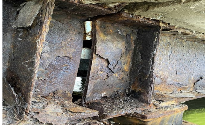
Deteriorated bridge structure
